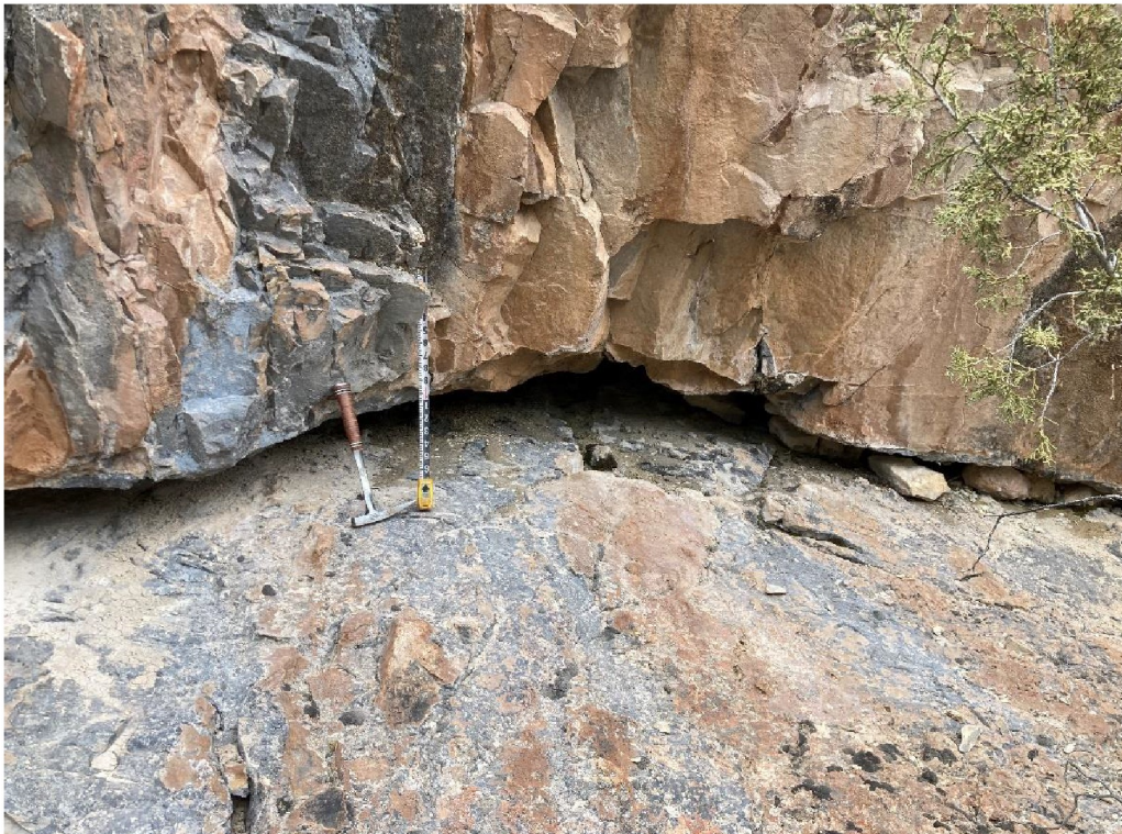
Photo 10: Location of exposed interbed of Photos 11 and 12 eroded back from outcrop face approximately 3 ft (4/14/23 Photo# 2024)
