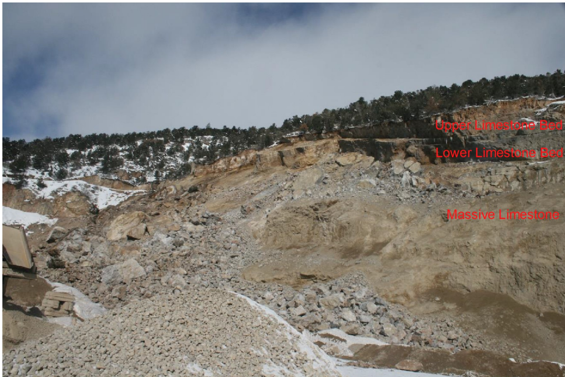
Photo 2: Overview of the January 18, 2023 ground event on the West Face. Rubble path and pile at left. The two upper units of the limestone are visible with bedding acting as the slide plane. (1/26/23 Photo# 0578)
